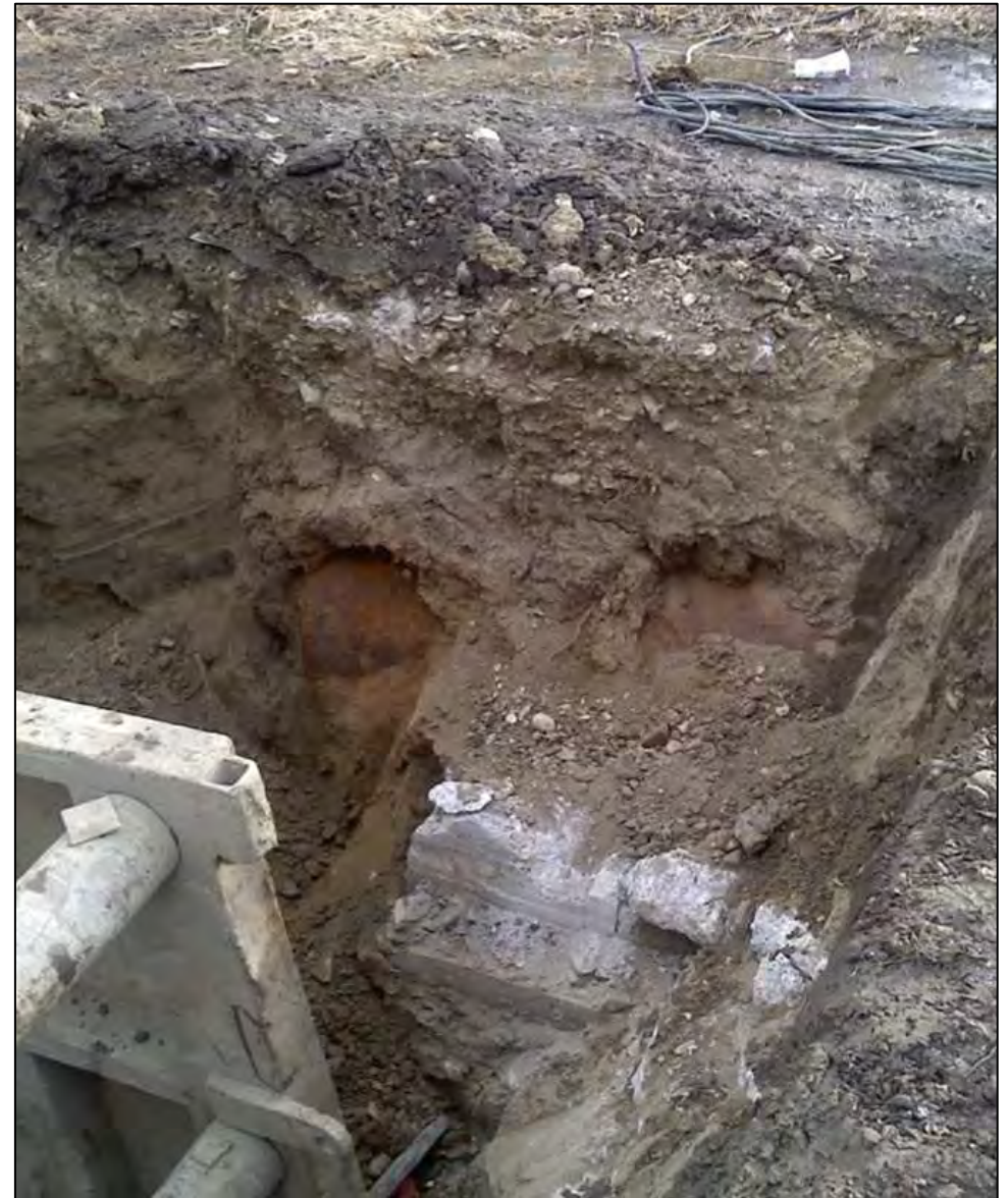
Abandoned underground storage tank discovered across the street from the elementary school during the water line project.
