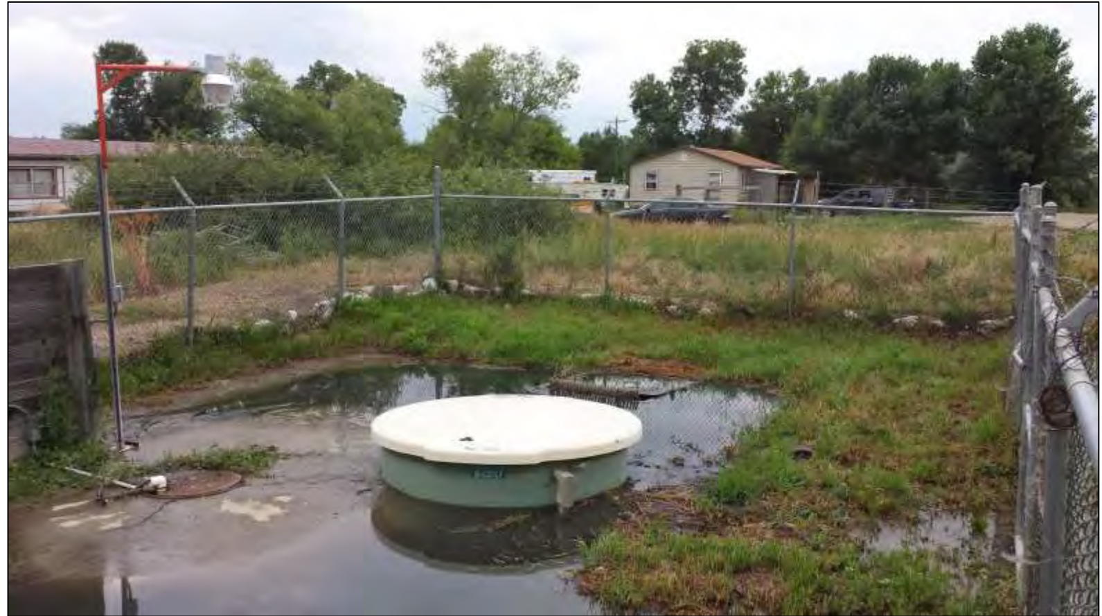
The Indian Health Service Hospital was closed for months when spring flooding swamped the public water supply lift station located in an old river oxbow.
