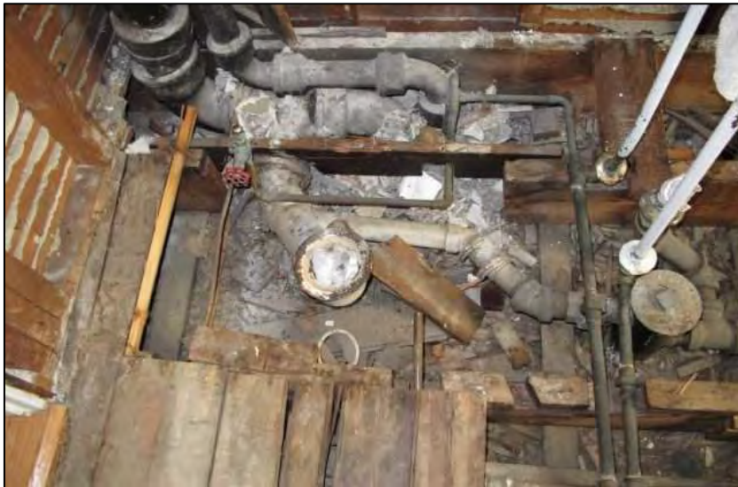
Failing home plumbing, including wells and septic systems
